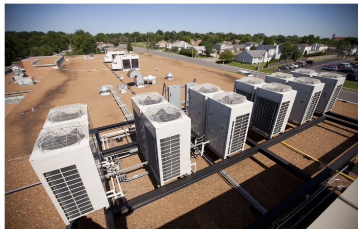
The VRV units pictured here helped provide the high school with energy efficiency equal to or greater than a geothermal system, with a significant reduction in classroom noise levels.
