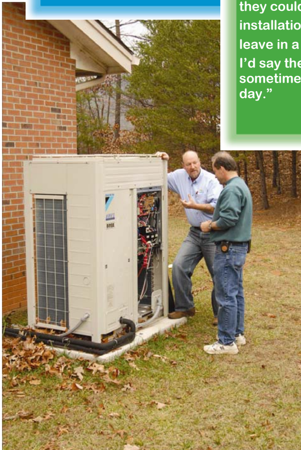
Daikin's VRV replaced a very large and expensive-to-run boiler that had to stay in operation from the end of September through May. In contrast, the VRV provides heating and cooling to individual areas, on demand, only when required.
