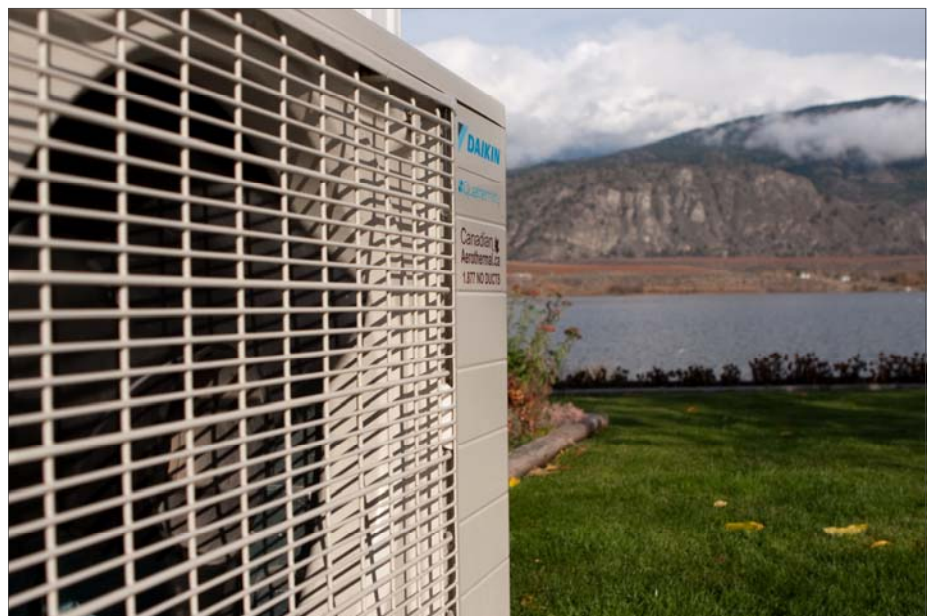
Jean Russell's home nestled in the Okanagan Valley in British Columbia, Canada, is now conditioned year round with Daikin's Quaternity™ heat pump system, which has the added functions of air purification and humidity control. The outdoor unit of the system is shown here.
